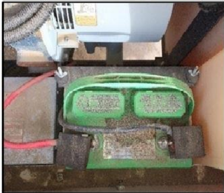
Original flooded lead acid battery
